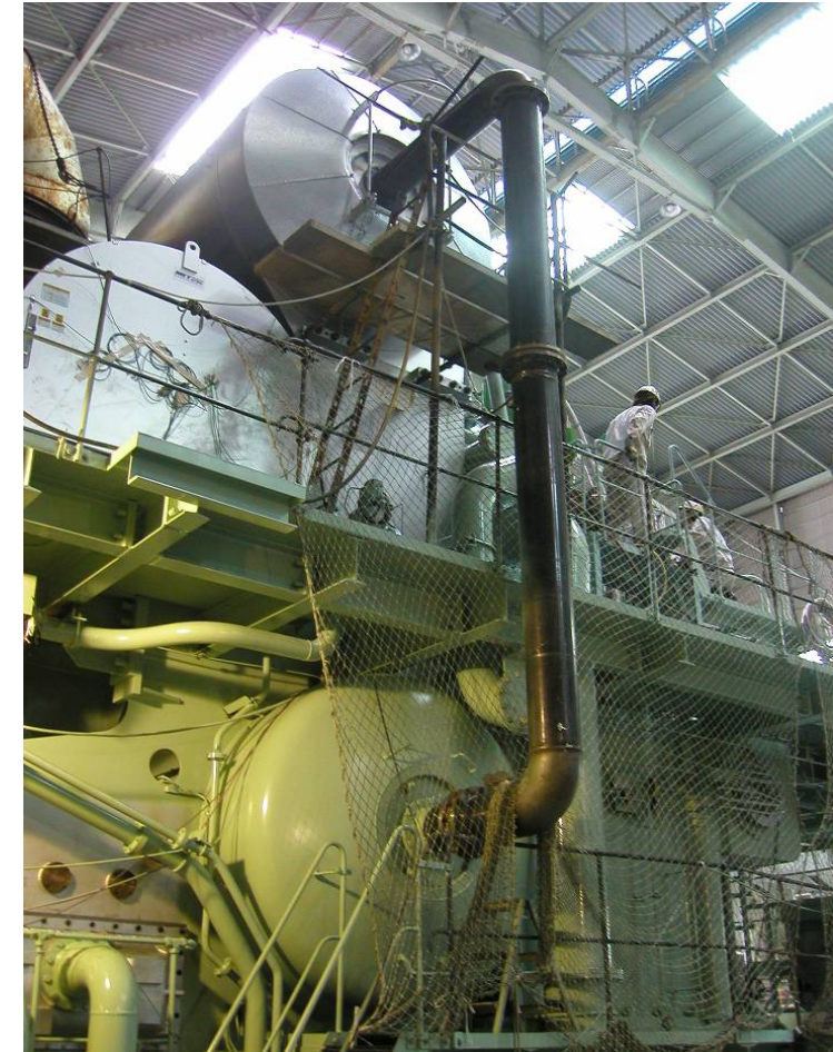
Fore and aft end bypass from the exhaust receiver to the scavenging air receiver
