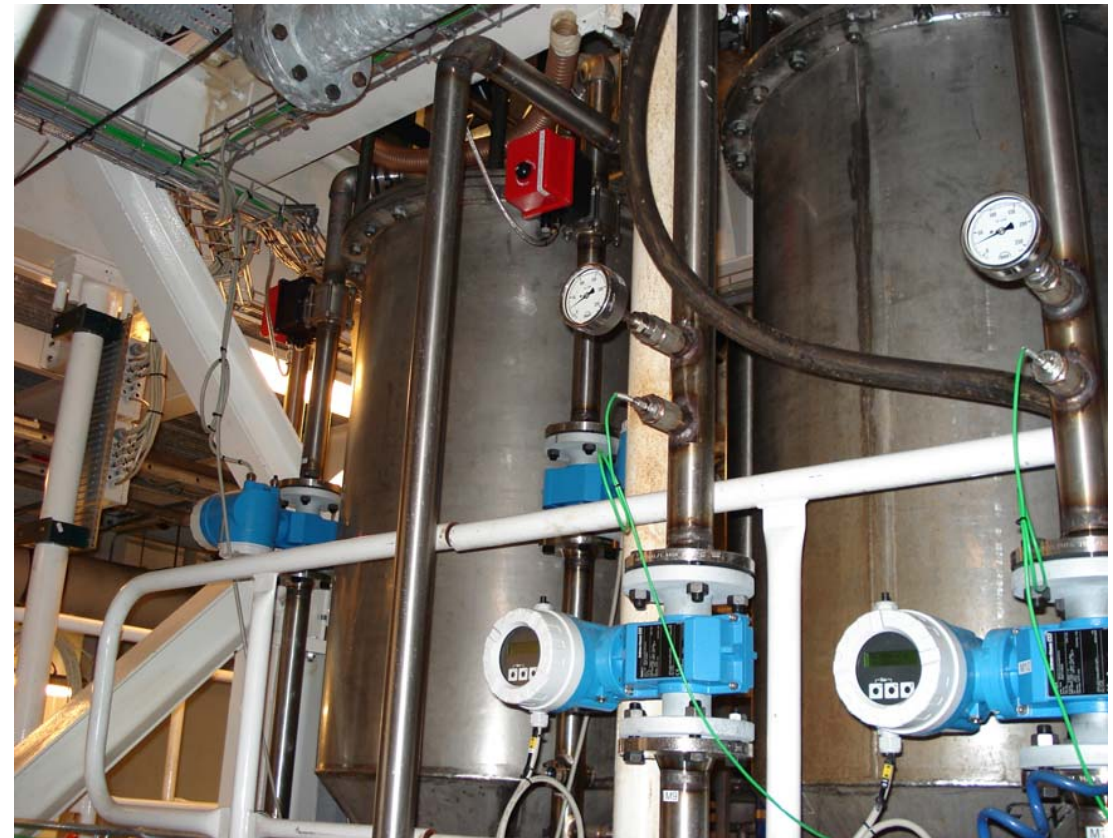
Water Treatment System
