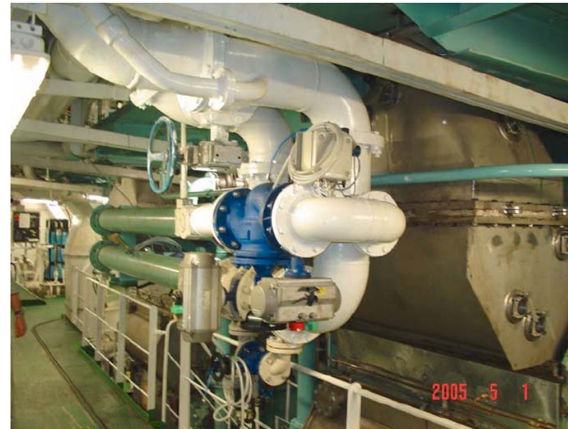
Changes on central cooling system
