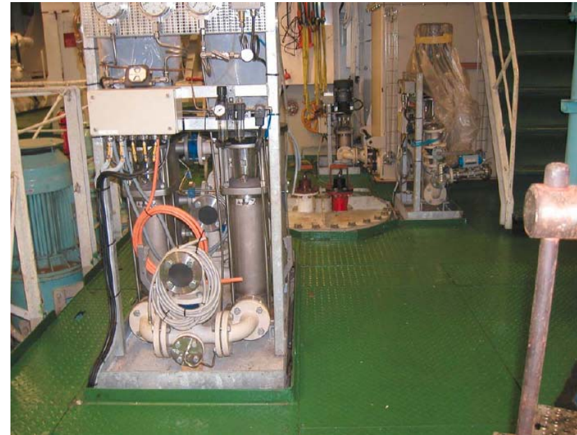
Sea water injection unit
