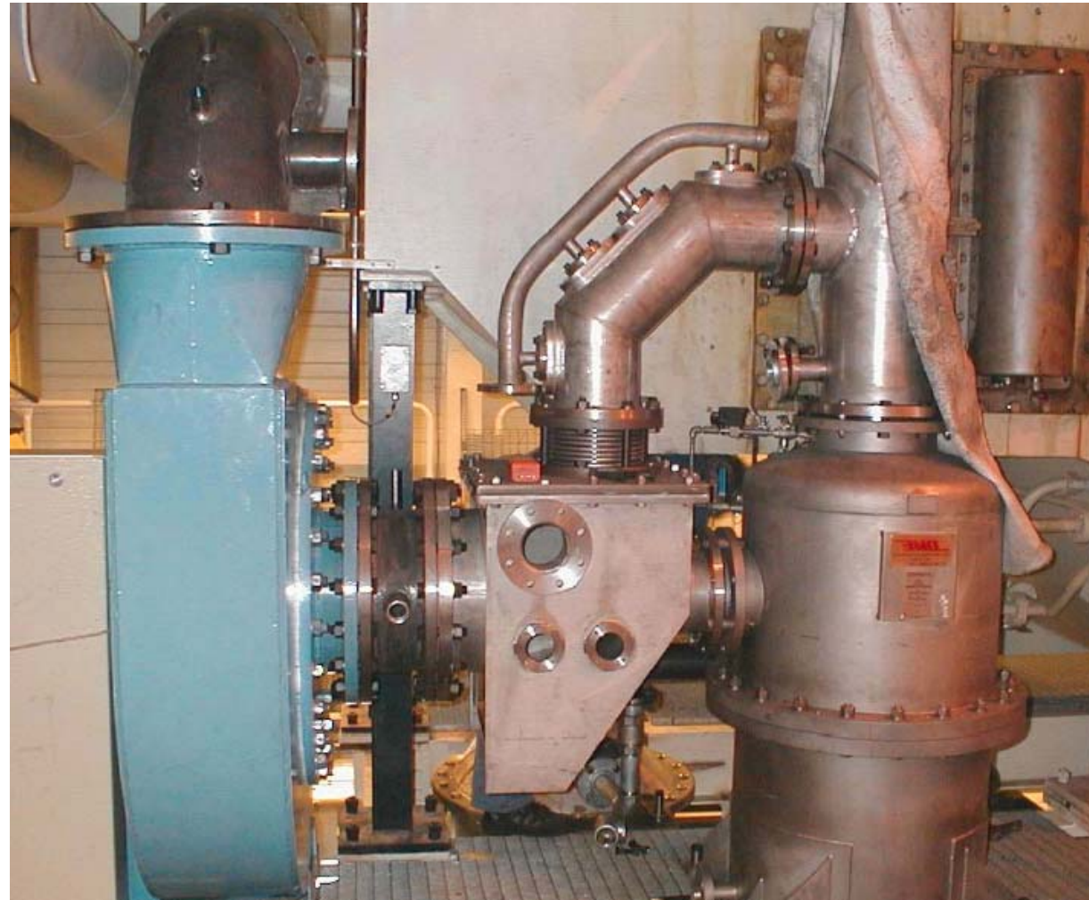
EGR scrubber and blower installed
