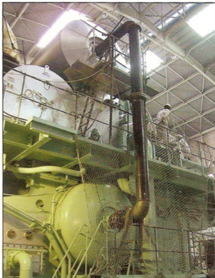
Fore and aft end bypass from the exhaust receiver to the scavenging air receiver used in task 4.2.
